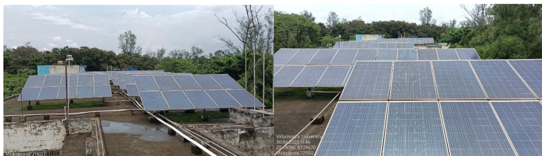
Plate 9: Solar Power panels
