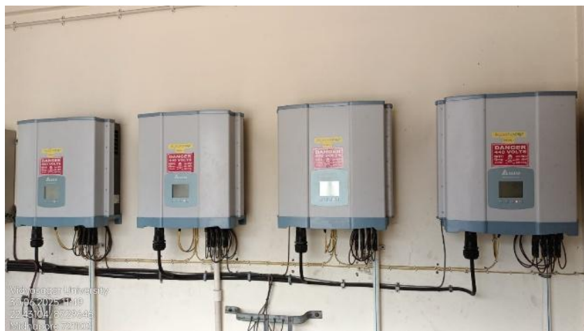
Plate 8: Solar Power Installation
